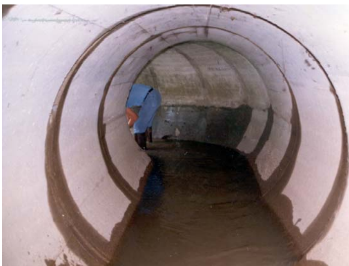
FIGURE 2: Typical Joint Infiltration in Non-Gasketed Storm Sewer
