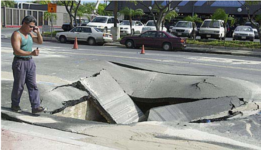
<FIGURE 1: Structural Failure From Loss of Fines>
