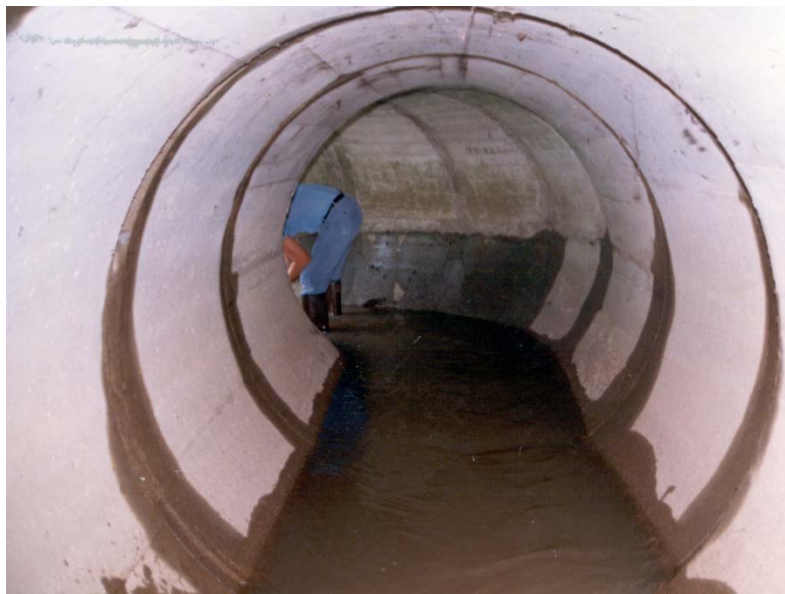
<FIGURE 2: Typical Joint Infiltration in Non-Gasketed Storm Sewer>
