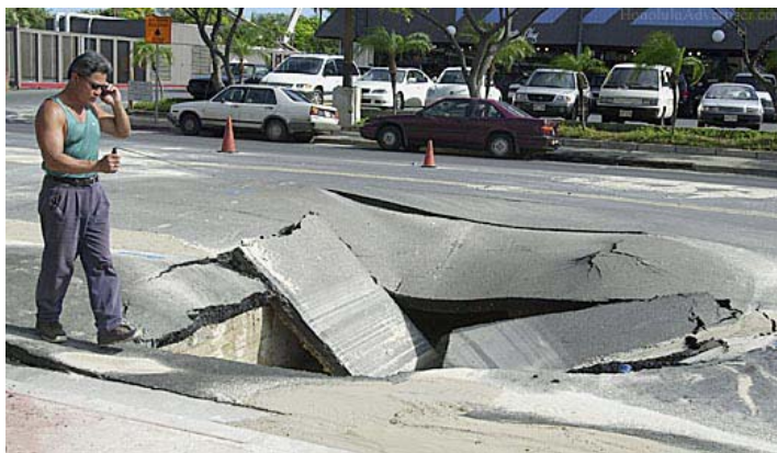
FIGURE 1: Structural Failure From Loss of Fines
