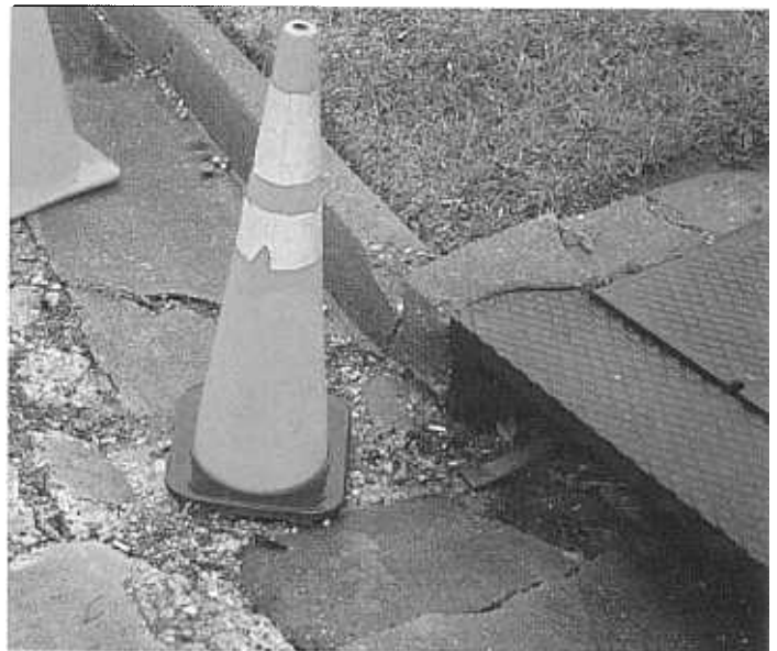
With 200 to 300 collapses around pipe and under 50 around structures per year, City Council appropriated an extra $467,000 for contract cave-in repairs like this one.
